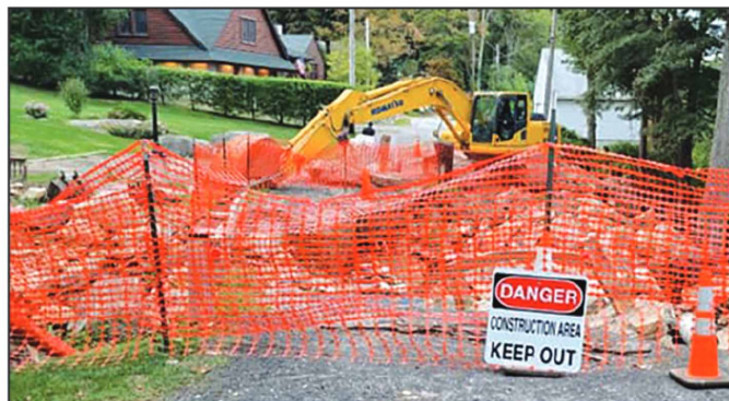
The absence of the bridge on Lakeview Drive near Whaley Lake has presented major obstacles for traffic and walkers for nine months, necessitating many large vehicles to turn around or to back down the road. For emergency responders, this leaves the entire community at risk in the event of failing to reach destinations on time.
